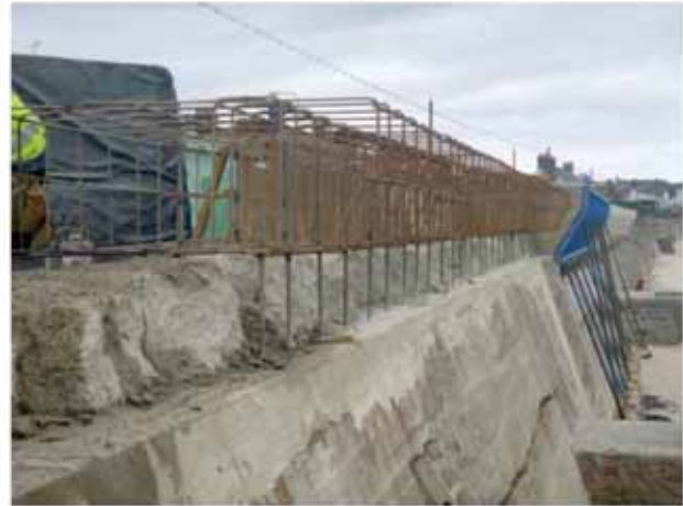
Figure 12. View of sequential construction of capping beam, raising the height and providing a recurve
