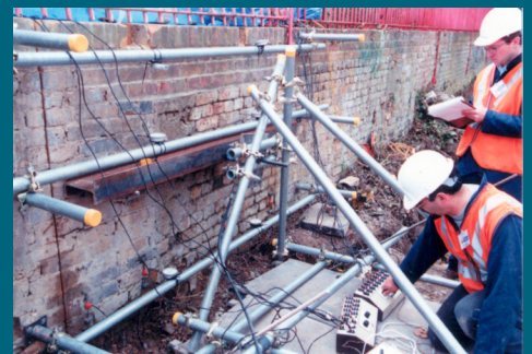
parapet walls can be strengthened at a fraction of the cost of traditional methods
