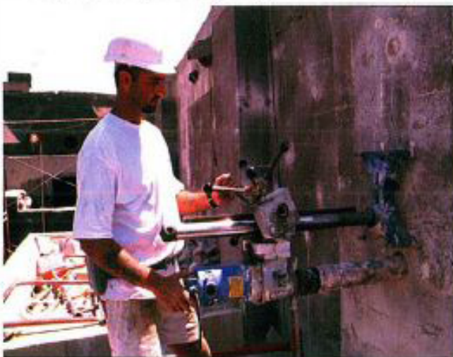
Non Percussive diamond drilling removes core into which a reinforcement will be installed.
