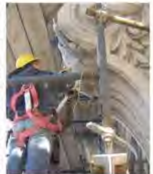
Grout being pumped into the terra cotta anchor assembly to engage and stabilize terra cotta units.
