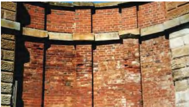
Damage to wingfall – note coloured cement render from 1930's and salt deposition caused by it.
