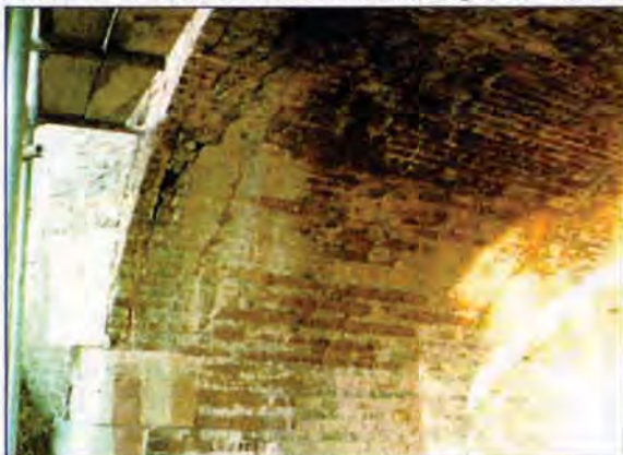
Typical damage to the soffit of the bridge
