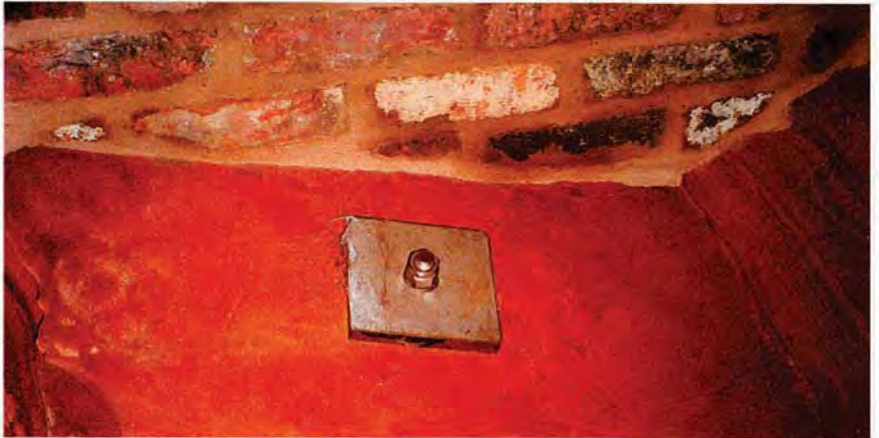
Roof bolt support to ballroom ceiling.
