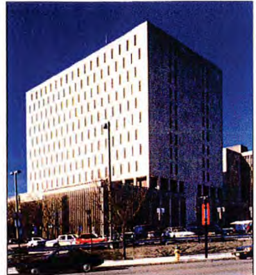
Limestone cladding of Essex County New Courts Building and Jail was one accident away from catastrophic failure. More than 20,000 Cintec anchors now prevent masonry's collapse.
