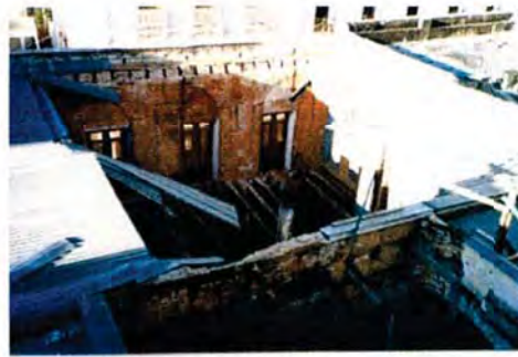
Real Audencia [post Earthquake] Puerto Rico
