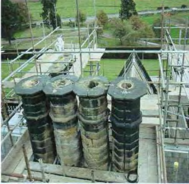
Partially missing ceramic liner ->
