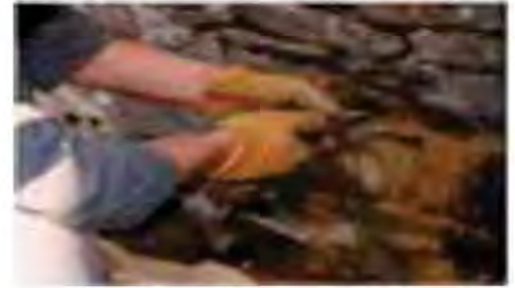
Insertion of 3m Cintec Anchor (left). Its inflation using cementitious grout, (above).
