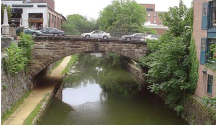
The Chesapeake & Ohio Canal flows under the stone masonry arch of the Wisconsin Avenue Bridge in the busy Georgetown area of Washington, DC. The towpath beside the canal serves as a footpath and recreation resource. The original wrought-iron railing dates back to 1831.
