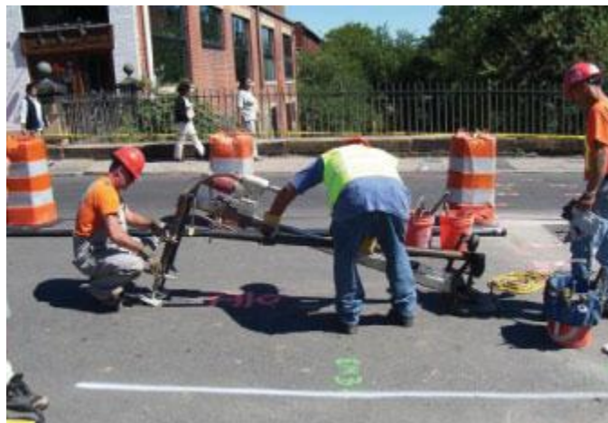
Workers bolt the drilling rig to the pavement on the bridge in preparation for drilling the 26 holes needed for the strengthening project.
