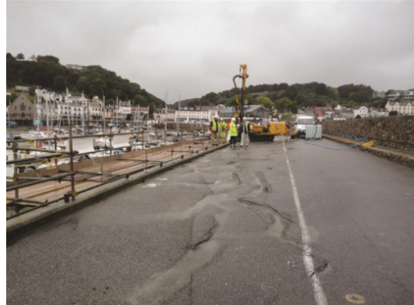
North Pier - cracks at deck level
