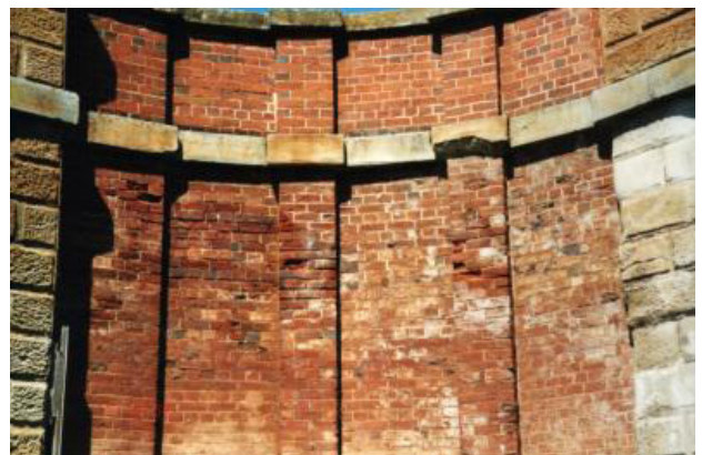
Damage to wingfall – note coloured cement render from 1930's and salt deposition caused by it.
