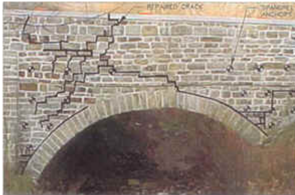
Figure 1: View of south spandrel wall showing the location of repaired cracks and remedial spandrel anchors.
