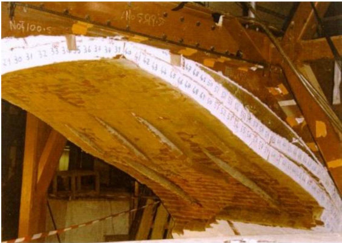
Figure 6: Arch after bottom ring fell away
