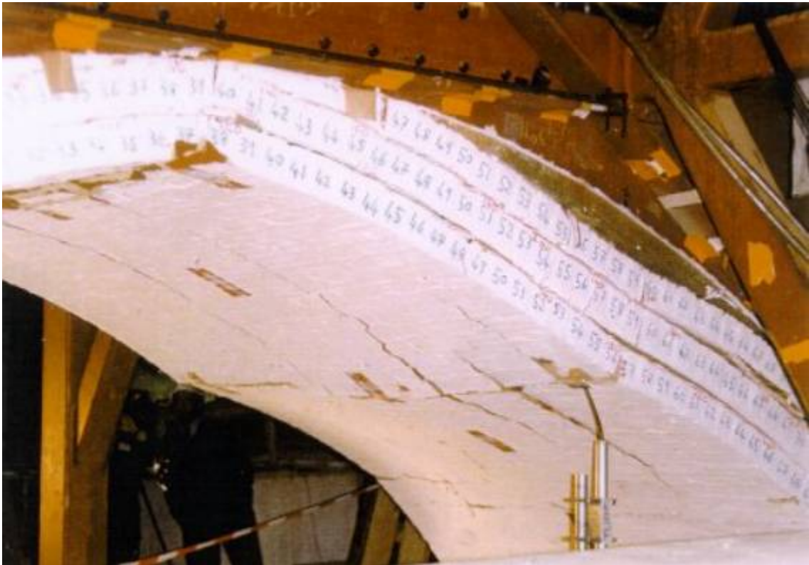
Figure 5: Arch just before bottom ring fell away
