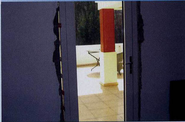
Figure 3 Door Perimeter Spalling
