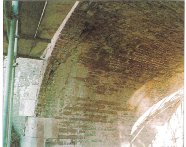
Typical damage to the soffit of the bridge
