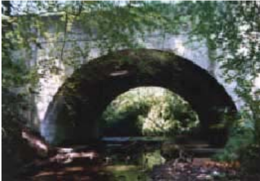
Figure 1. Elevation of Cascade Bridge. The structure has a clear span of 10.5m and a width of approximately 12.5m. The bridge is entirely of brick construction apart from a concrete slab footpath on one side. The structure provides for a single lane carriageway of width 9.5m. The structure spans a small stream with large seasonal flow differences. The structure is presently 175 years old.
