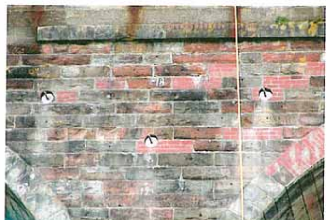
Inflated pipe anchors (Holes subsequently plugged and hidden).
